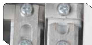
Provision for Isolation of Neutral link to Carry out Insulation Test
