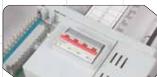
Neutral and Earth link are Completely Shrouded
